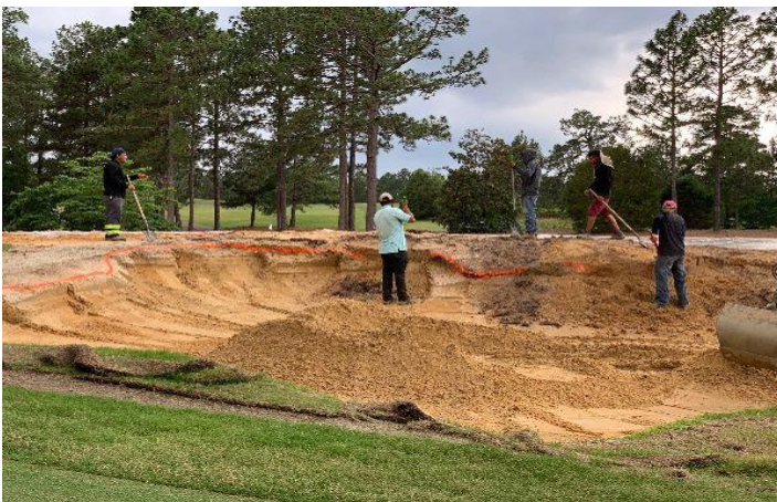
Left greenside bunker #18
