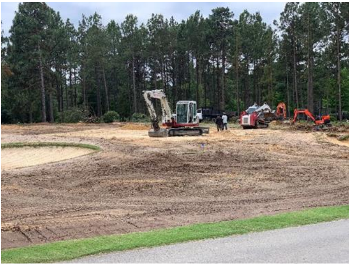
The short game area has been stripped of all grass. The new green and bunkers will be repositioned and shaped in the coming days.
